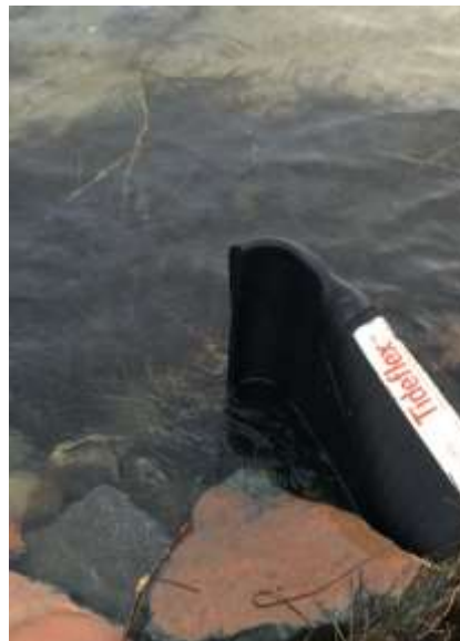
The duckbill valve installed at Village Bay Close. Credit: Rob Mackenzie.
