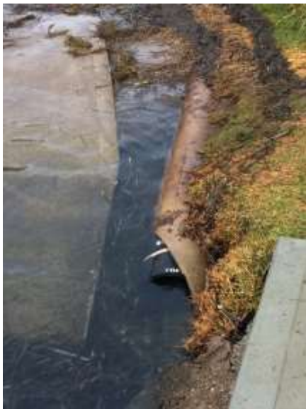
The 'Checkmate' valve installed at Marks Parade. Credit: Rob Mackenzie.
